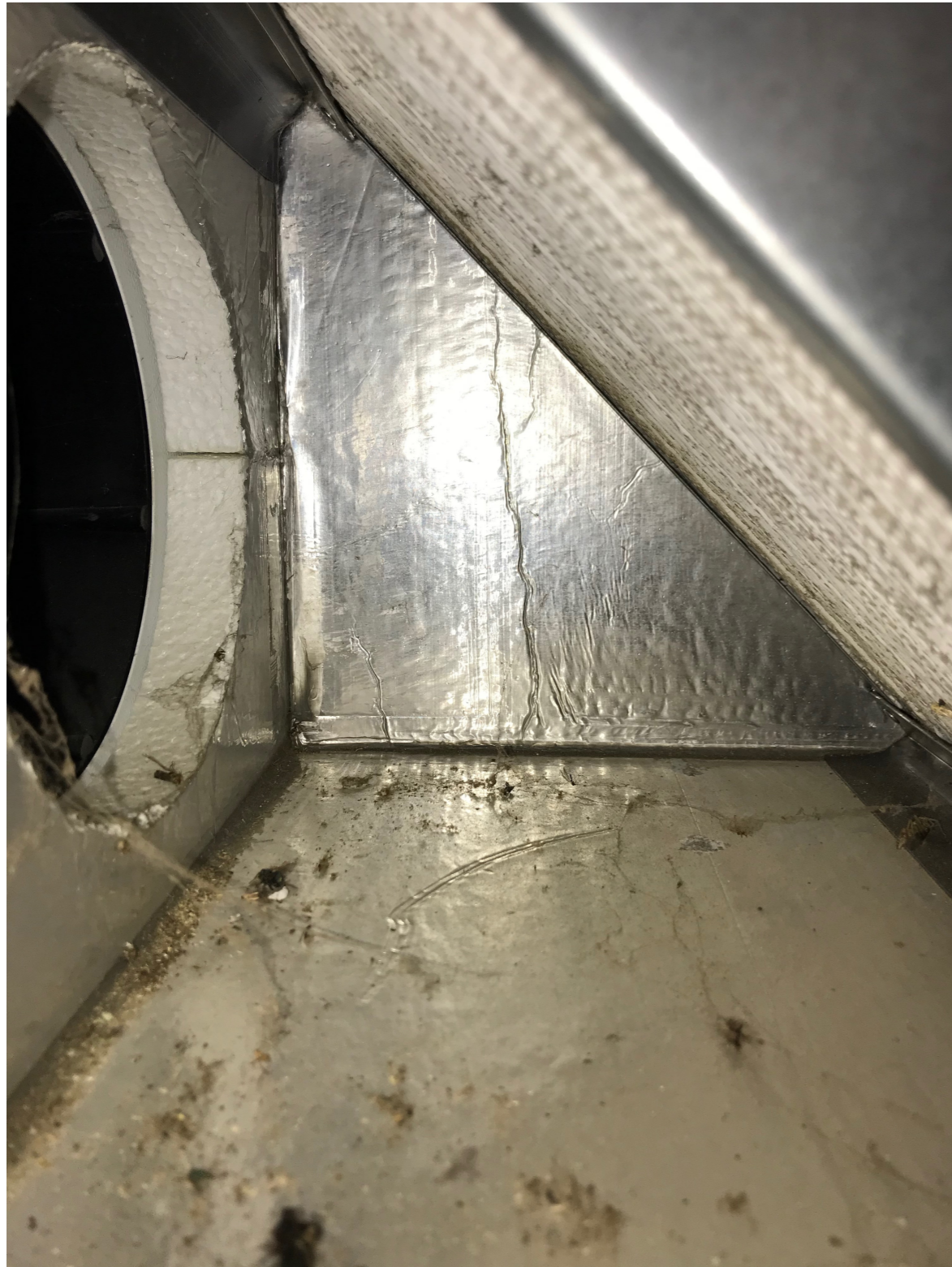
Interior of the ventilator - intake chamber
